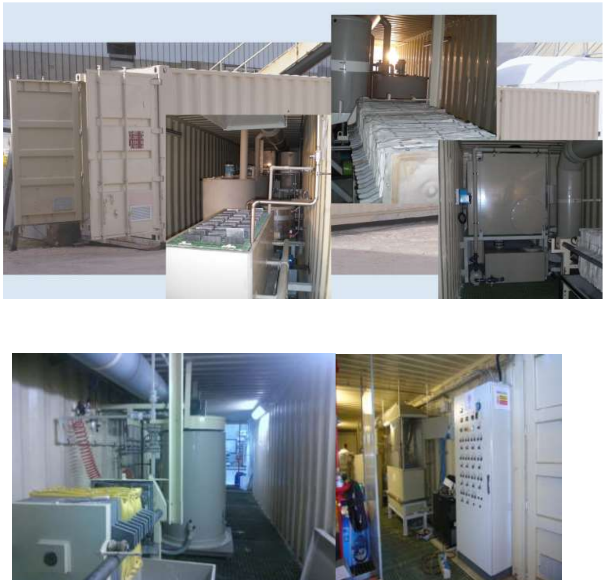
Fig. 6 Mobile plant from Hydroweee Project.
